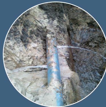
Leaks on pipe in rural area. Serious leakage of 400,000 m 3 /y. It did not surface but was found when sectioning the network and by manual leak detection.
