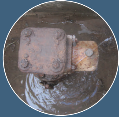
Leaking valve in valve chamber. Leaking 500 m 3 /y. Regular valve surveys would minimize the run time of such leaks.
