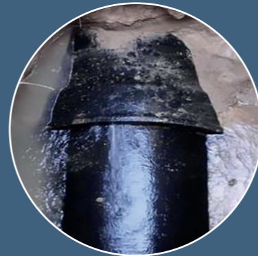
Buried leak that does not surface. Leaking 2,500 m 3 /y. Active leakage control would lead to shorter run time.
